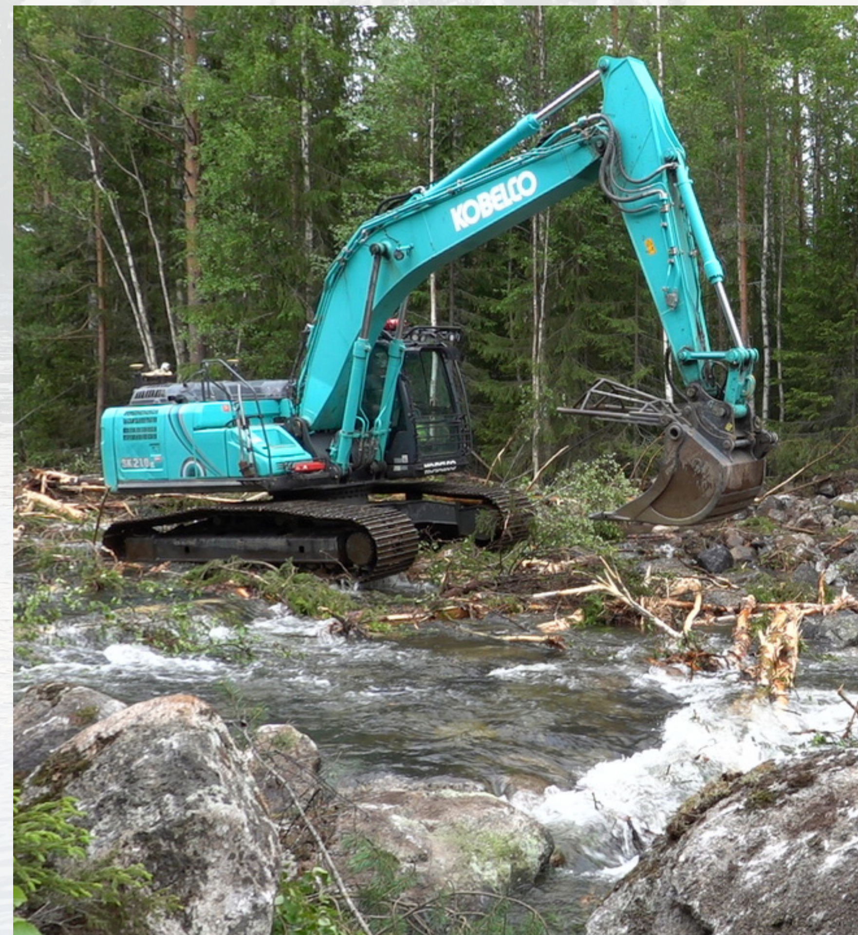
Excavator working in Agnelån. Careful planning before and on-site during the excavation work is essential for the best possible results.
